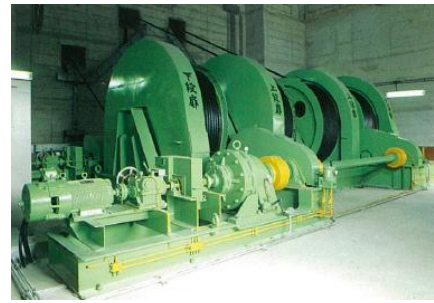
Selective water intake gate opening and closing equipment
