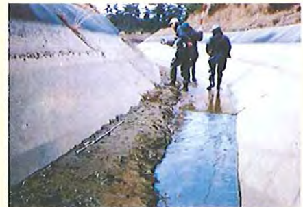
Sedimentation in the canal
