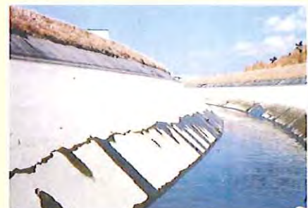
Cracks and Leak in the canal
